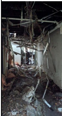
Damage after the fire
